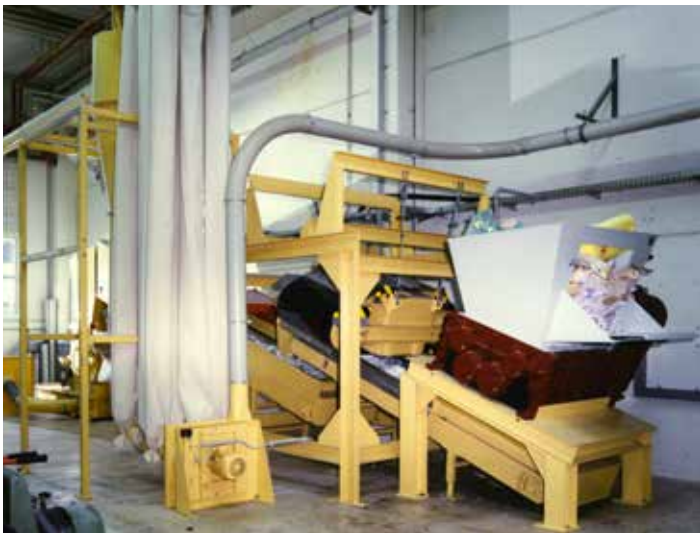
Thousands of tonnes of foam are processed in the new recycling plant in Linz (Austria).
